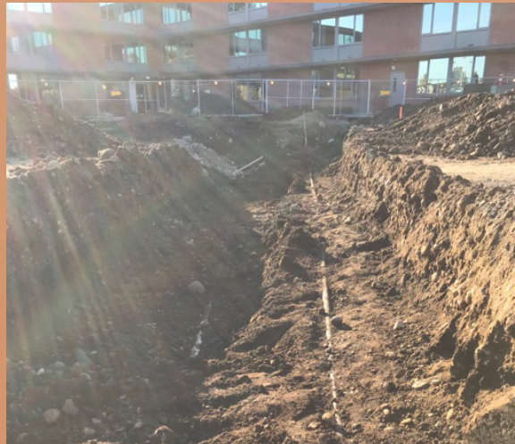
Old gas and water lines being removed from under the Memory Care building
