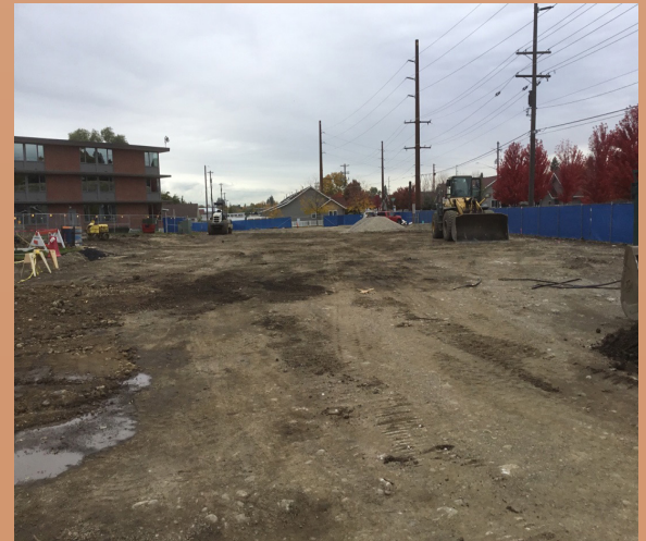
The construction site has been graded and is ready for building staking
