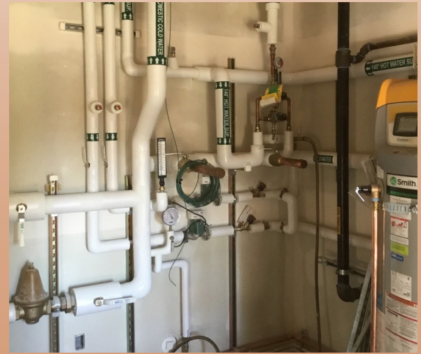
KC Charles has done a great job installing piping in the water mechanical room
