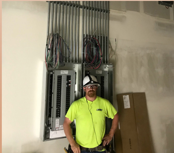
Kramer with Summit Electric displaying his electrical panel and conduit rack rough-in craftsmanship
